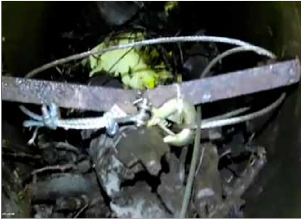
View of the metal grate and trapped blockage.
