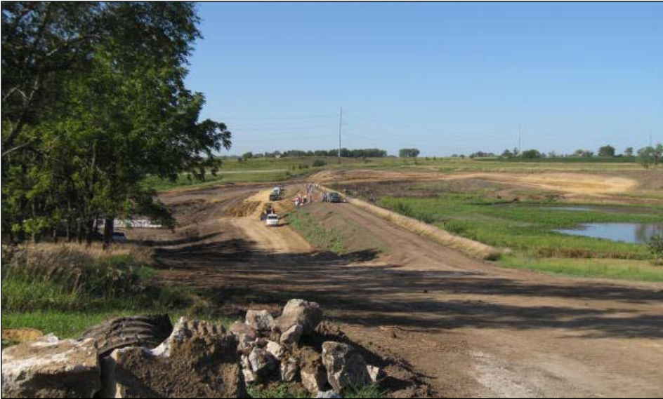
Taken in early September, this photo shows work progressing on the rehab of Wilson Creek 8-H.
