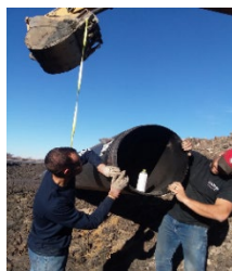
Left: LBBNRD employees guide a tube into place on a recent maintenance project.
